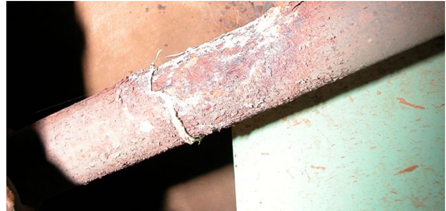
A close up view of acidic condensate damage on a pipe exterior.
