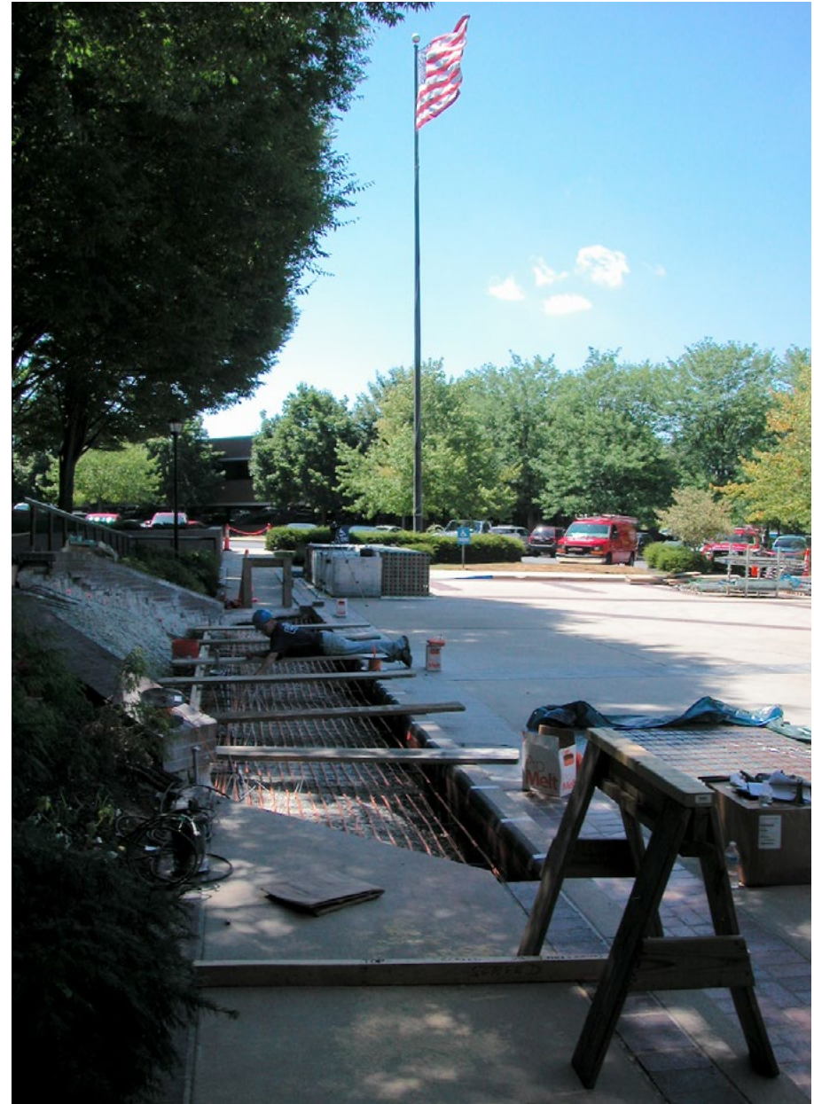
ProMelt cables are installed on the lower sidewalk.
