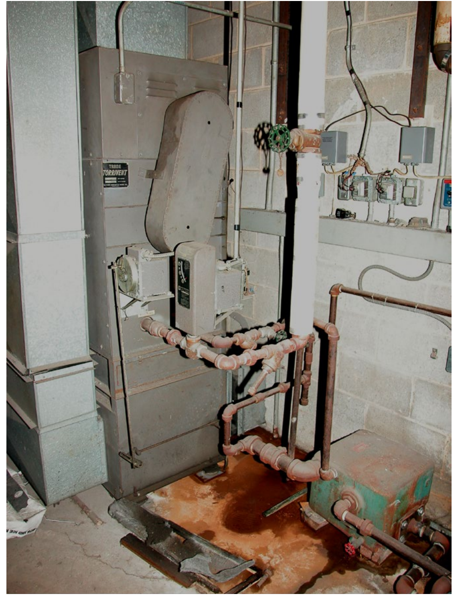
The old steam hydro-air unit.
