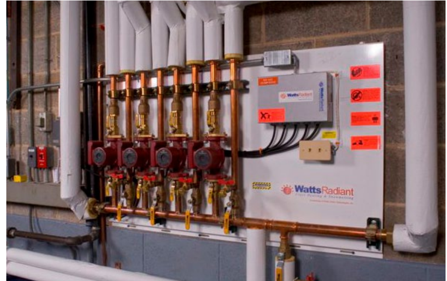
The Watts Hydronex distribution control panel.
