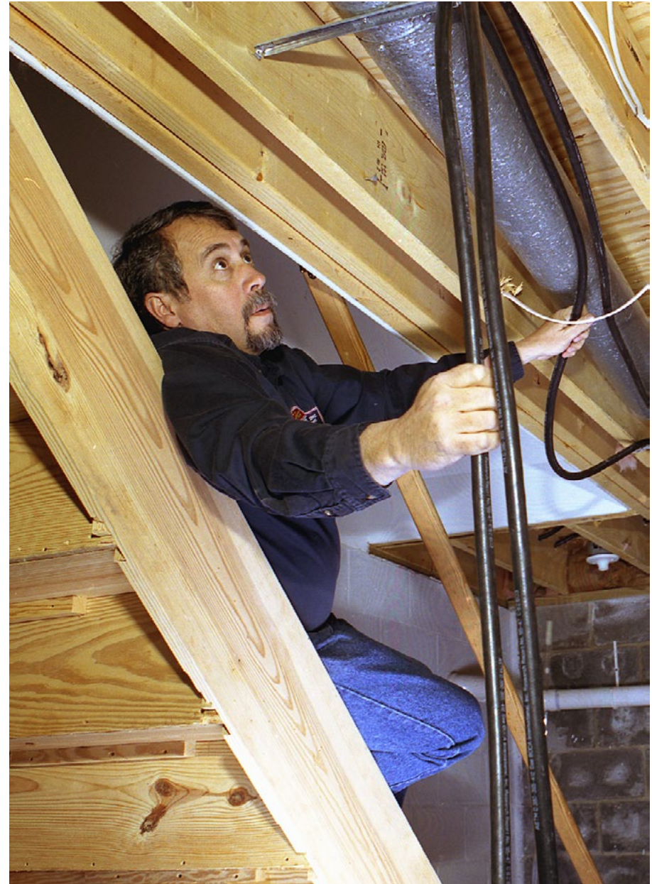
Dave Yates threads Onix tubing through the joist bay. Photo by John Herr.
