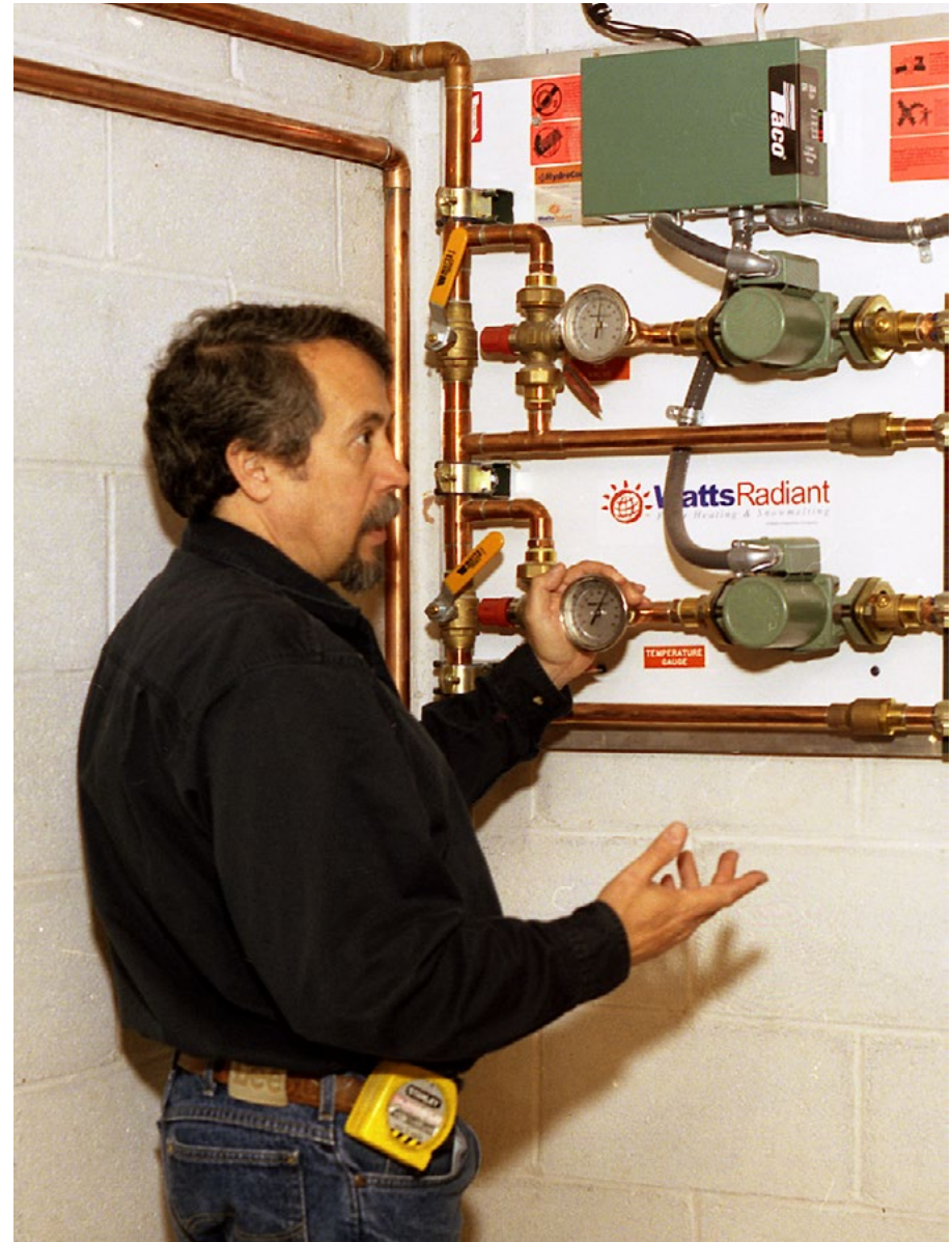
Dave Yates checks over the Watts control panel. Photo by John Herr.
