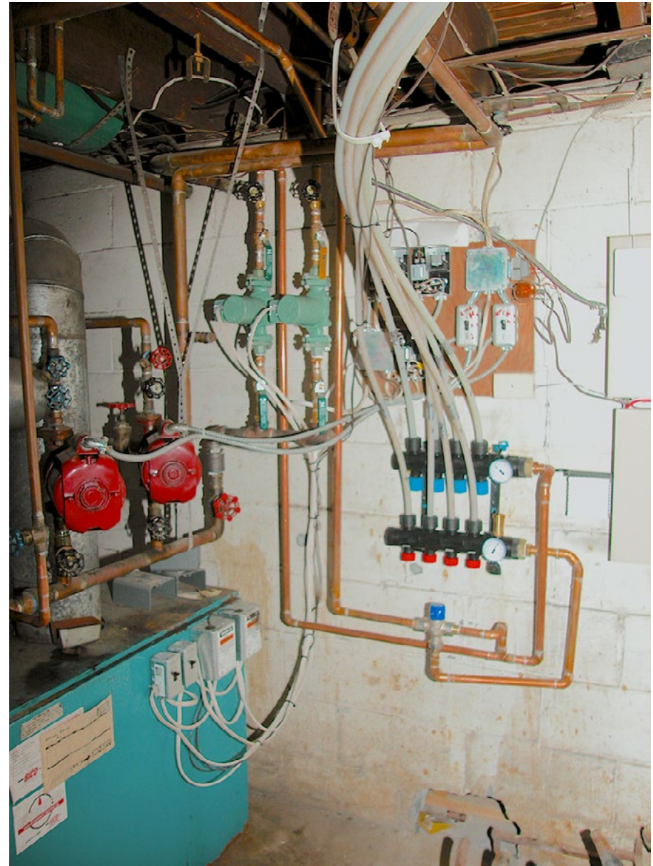
This mechanical room shows lots of room here for dramatic improvement!
