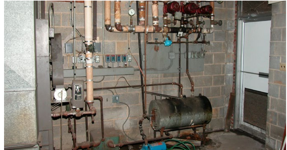
Pictured here is the steam hydro-air on the left; steam condensate receiver/pump and freed-water tank at the bottom right; and hot water distribution piping and circulators at the top right.
