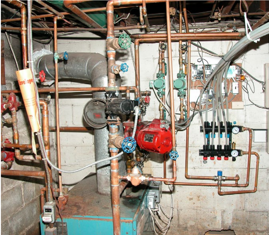
Hydronic mayhem, layer upon layer.
