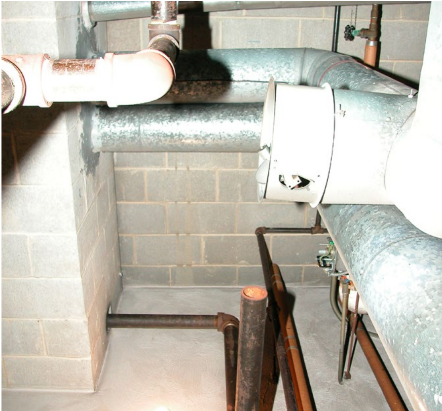
Pipe corrosion from acidic condensate dripping down from open pipe connected to chimney base.
