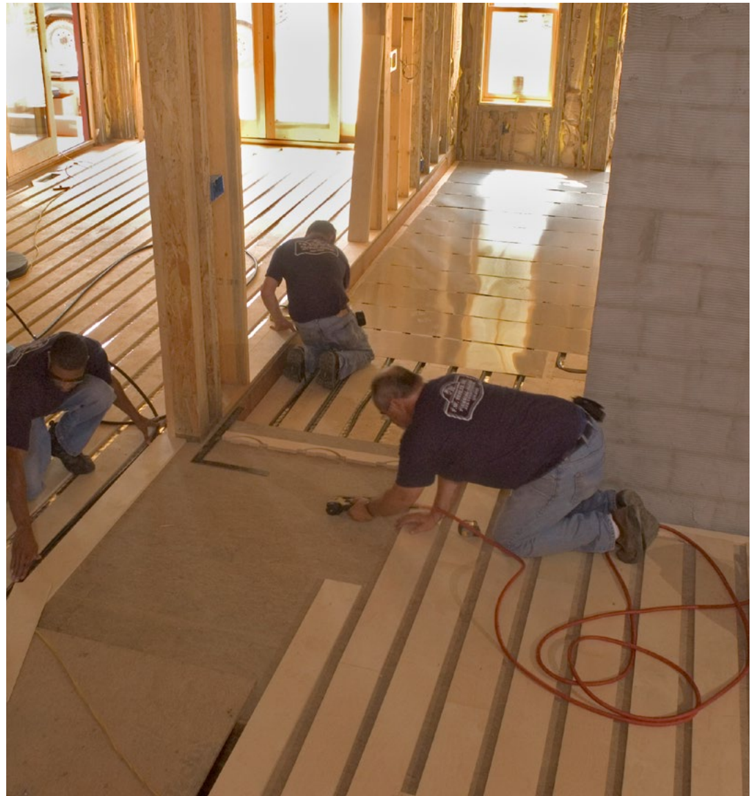
The Behler crew installs Watts SubRay panels, Onix tubing and heat transfer plates.
