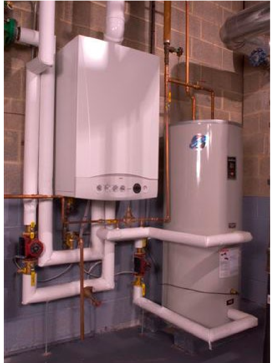
The Laars modcon boiler and Bradford White indirect water heater.
