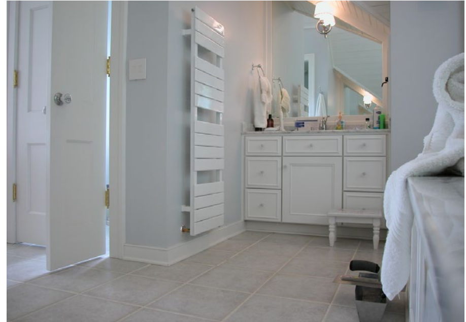
Master bathroom combi-towel warmer and radiant flat panel radiator to supplement heating.
