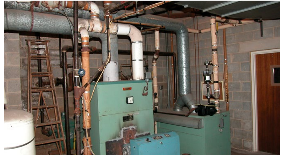
Pictured is the steam boiler on left with the hot water boiler on right.
