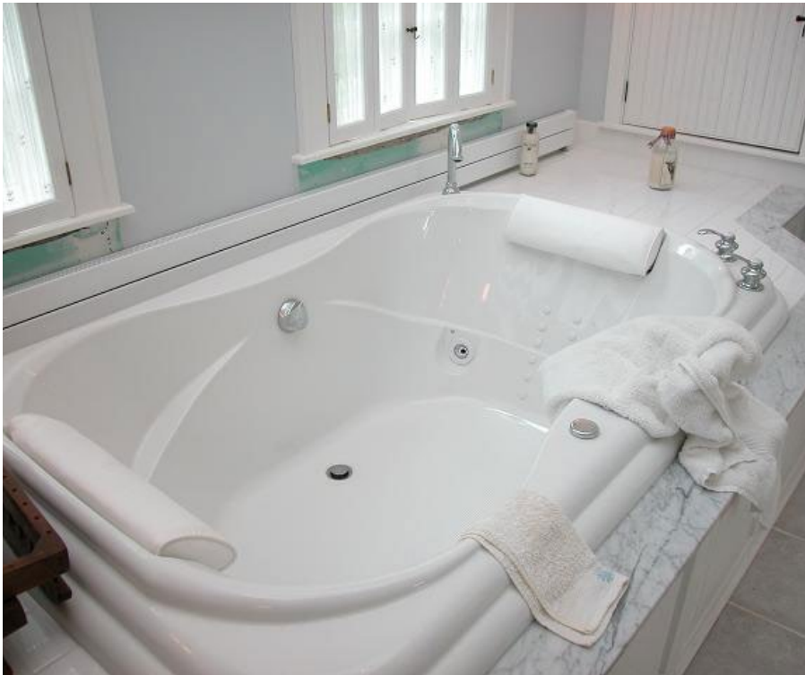
The flat panel radiator to offset chill from adjacent window and supplement heating.
