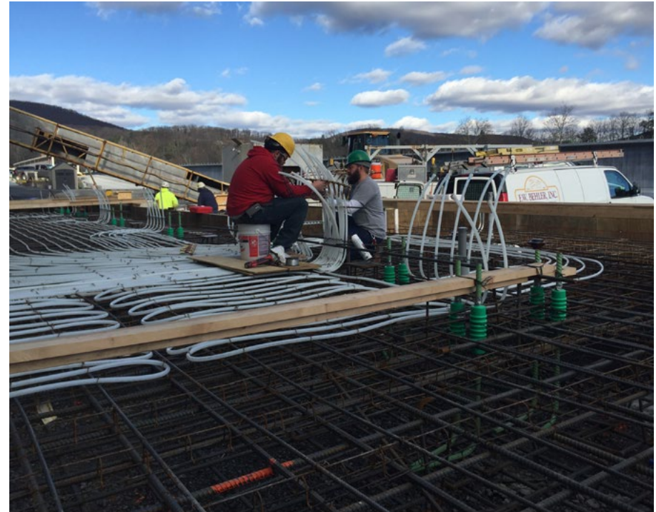
Installing a test manifold while working atop the three foot thick rebar assembly.
