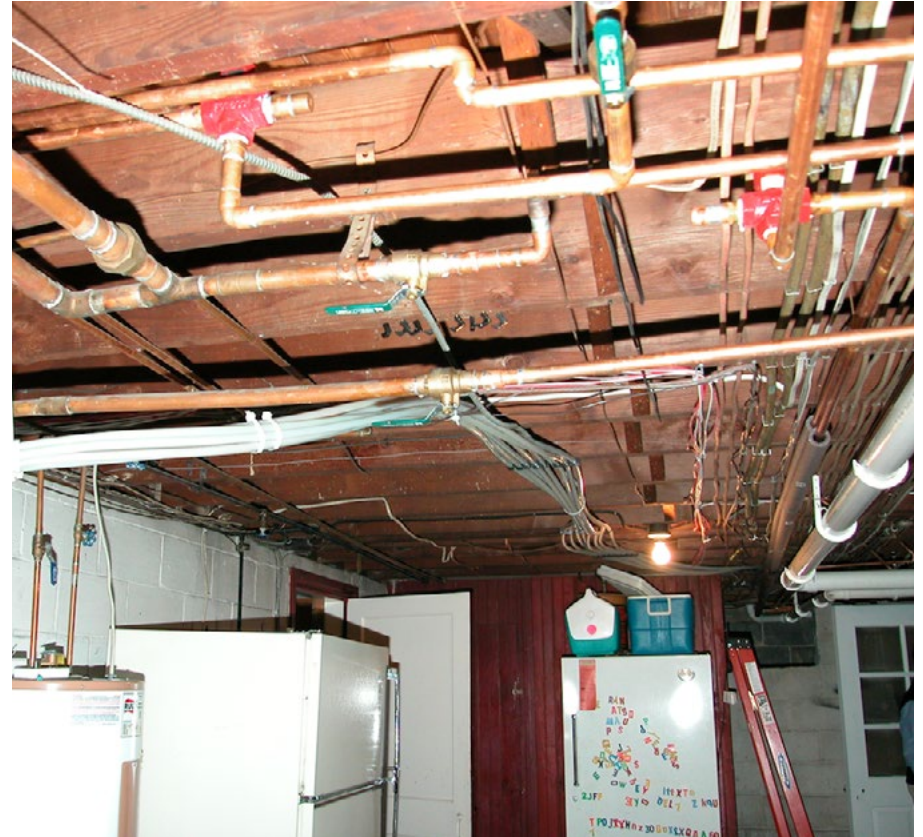
Workmanship lacking: PEX leader lengths are too long, poorly supported and not insulated.
