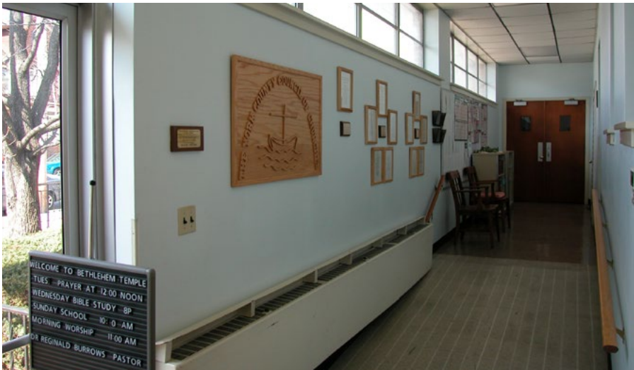
A convector in a classroom hallway.
