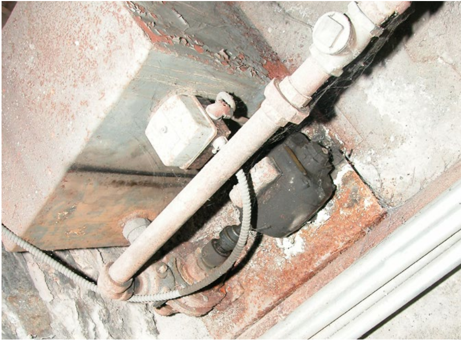
Pipe corrosion from acidic condensate dripping down from open pipe connected to chimney base.
