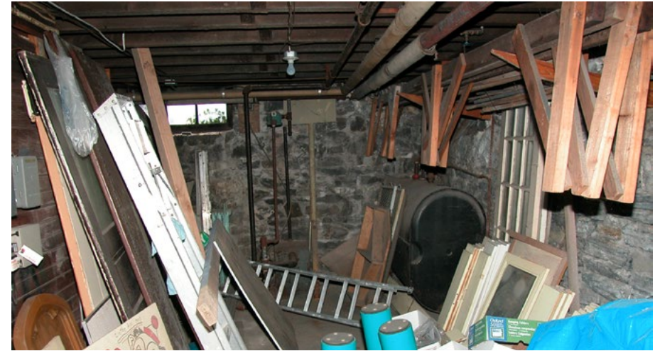
Where's Waldo? A remote antique condensate pump at the far end of the storage room, adjacent to an abandoned oil tank.
