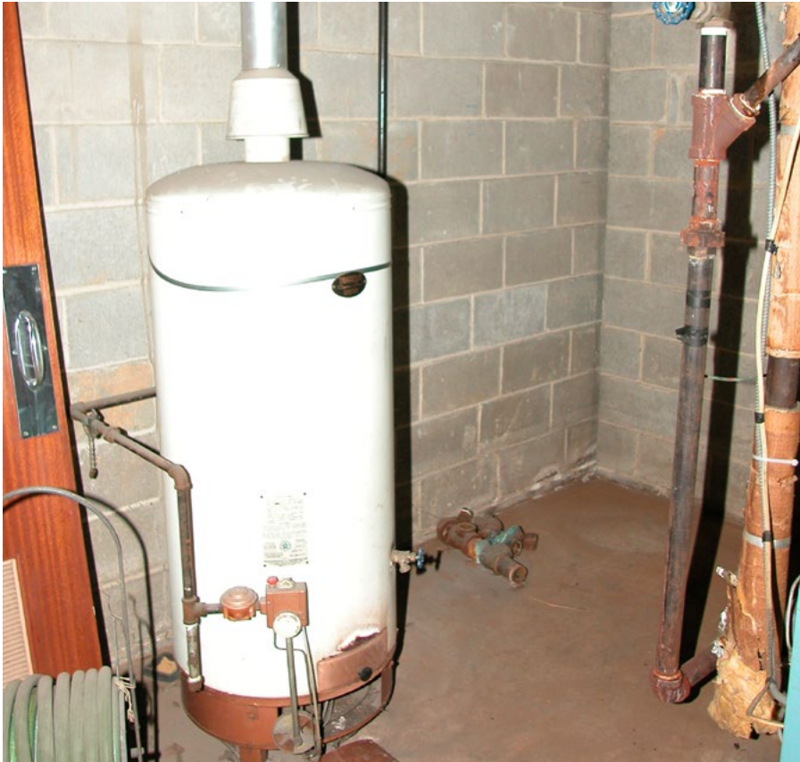
The old, tired water heater.
