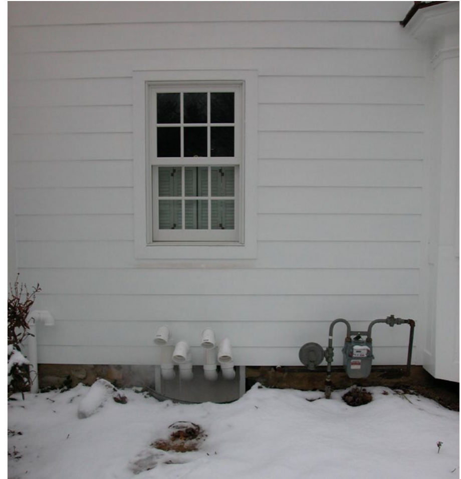
The original vent terminations.
