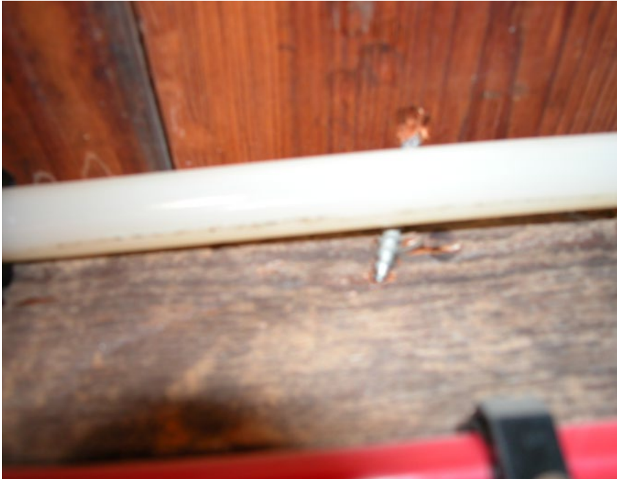
PEX installed in contact with sharp screw threads.
