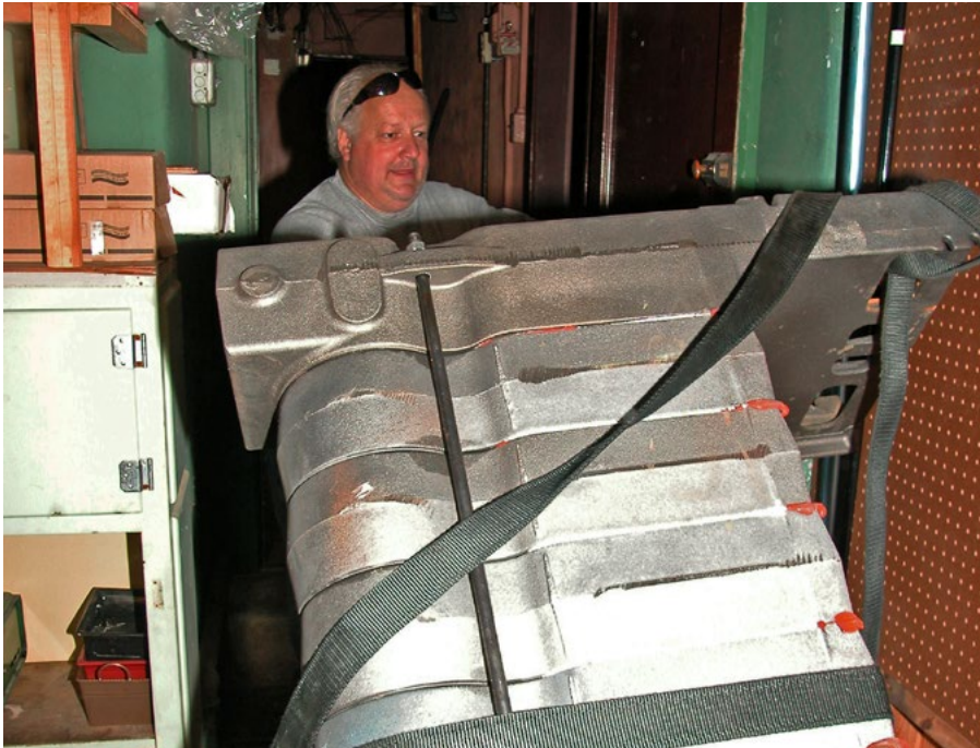
Les Scrivens of Thomas Somerville goes above and beyond while helping move the Weil McClain steam boiler into the mechanical room.
