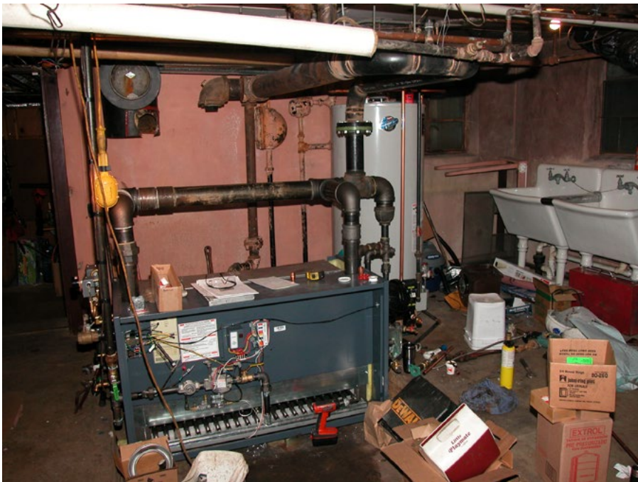
The new steam header and piping joins to the old system piping.
