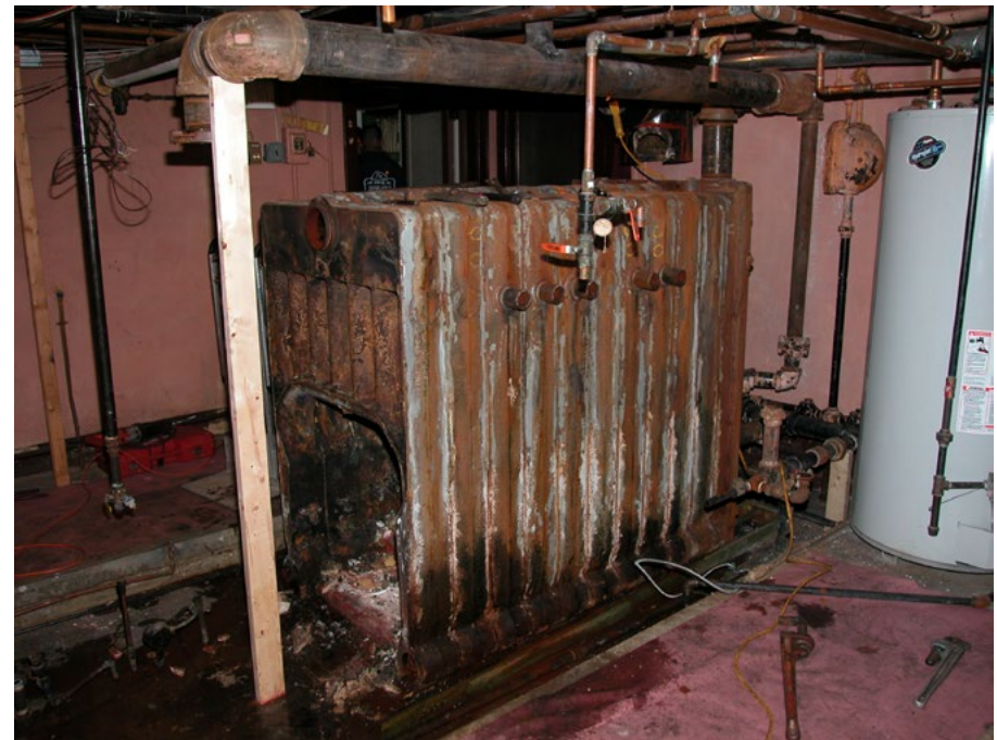
The existing boiler was grossly oversized.
