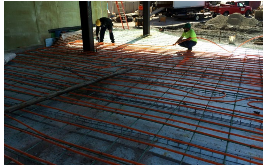
In all, 14 miles of 3/4-inch Watts Radiant RadiantPEX+ with a 50% glycol mix were installed once the project was completed.
