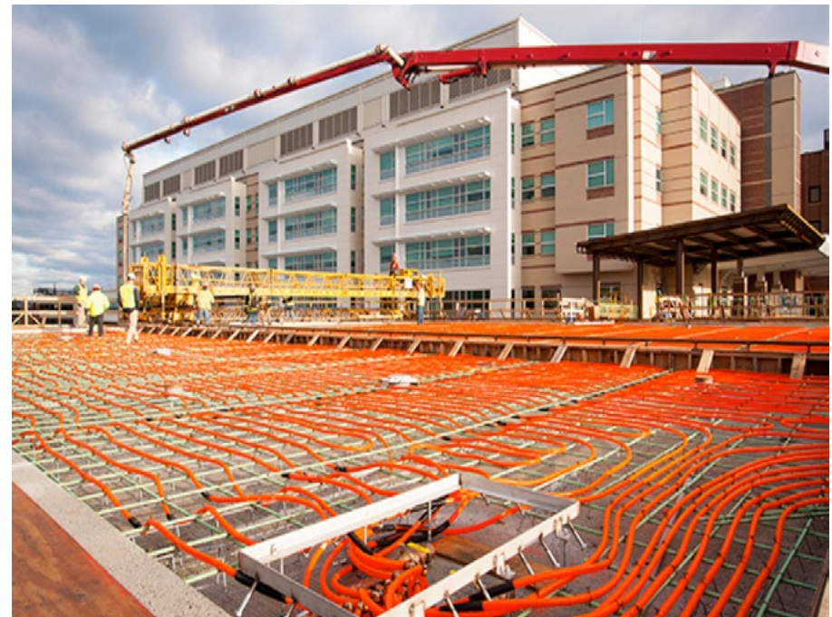
Fourteen miles of 3/4-inch Watts Radiant RadiantPEX+ with a 50% glycol mix were installed once the project was completed.
