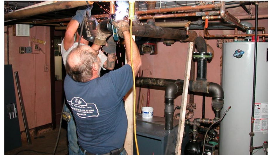
Scott Barnett with F. W. Behler works with the welder building the new steam piping on-site.
