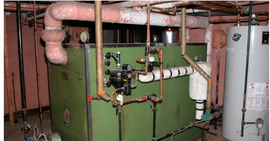
We were awarded the installation of a large commercial-sized cast iron steam boiler for a very large home built back when coal was king.
