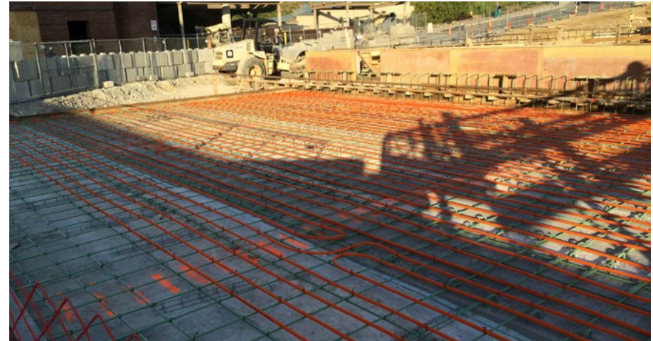
More than 16,000 lineal feet of 3/4-inch Watts Radiant RadiantPEX+ tubing was installed before the helipad's cement surface was poured.
