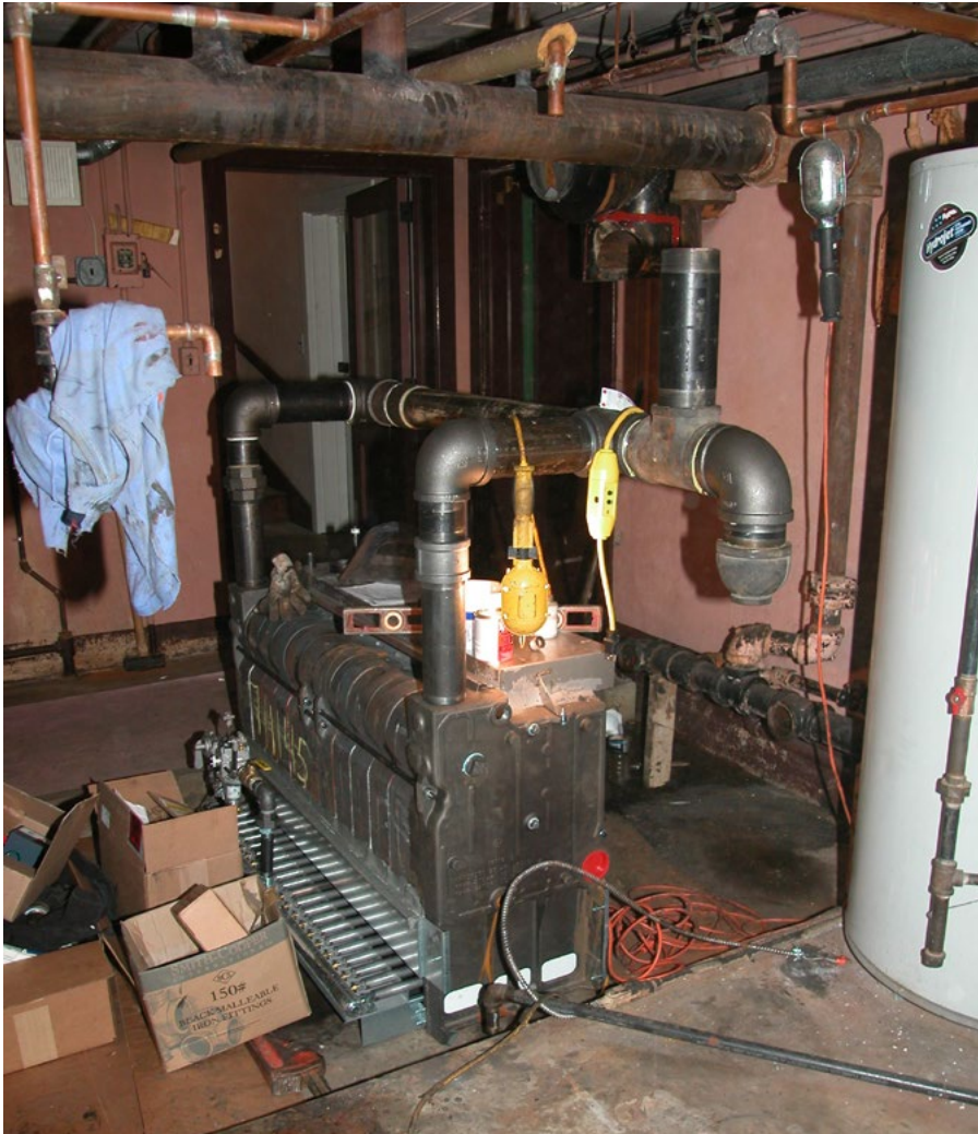
The new steam header and piping joins to the old system piping.
